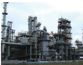
Sulfur-free gasoline production units
