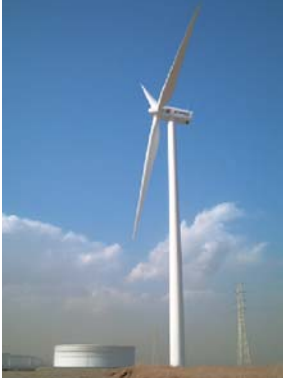
Wind power generation facilities Opened in March 2005, at the Kashima Oil Refinery. Japan Energy Group's second such facility.
