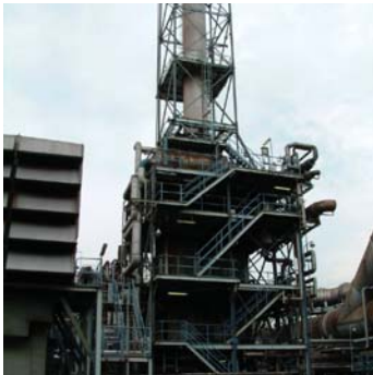
Boiler waste heat recovery equipment
